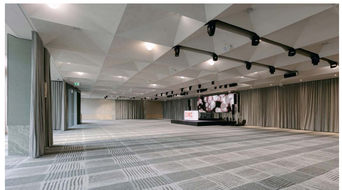
Zinc's new sophisticated AV system design with dbTechnologies achieves even sound coverage throughout the venue while preserving its clean visual lines.
