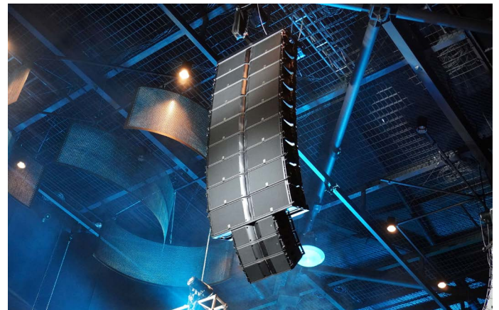
An array of L-Acoustics K2 and Kara II in the Great Hall of the Brisbane Convention & Exhibition Centre.
