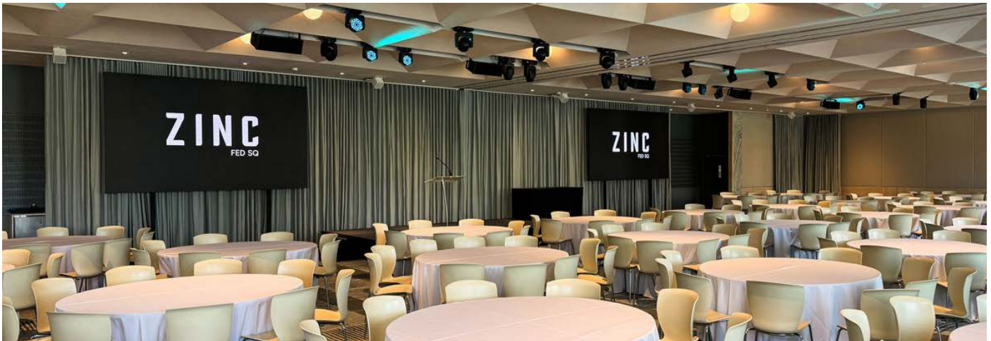
Sound-absorbing panels, drapes, and sound-dampening paint have been applied to the ceiling baffles to resolve the noise issues that previously hindered the space's audio clarity.
